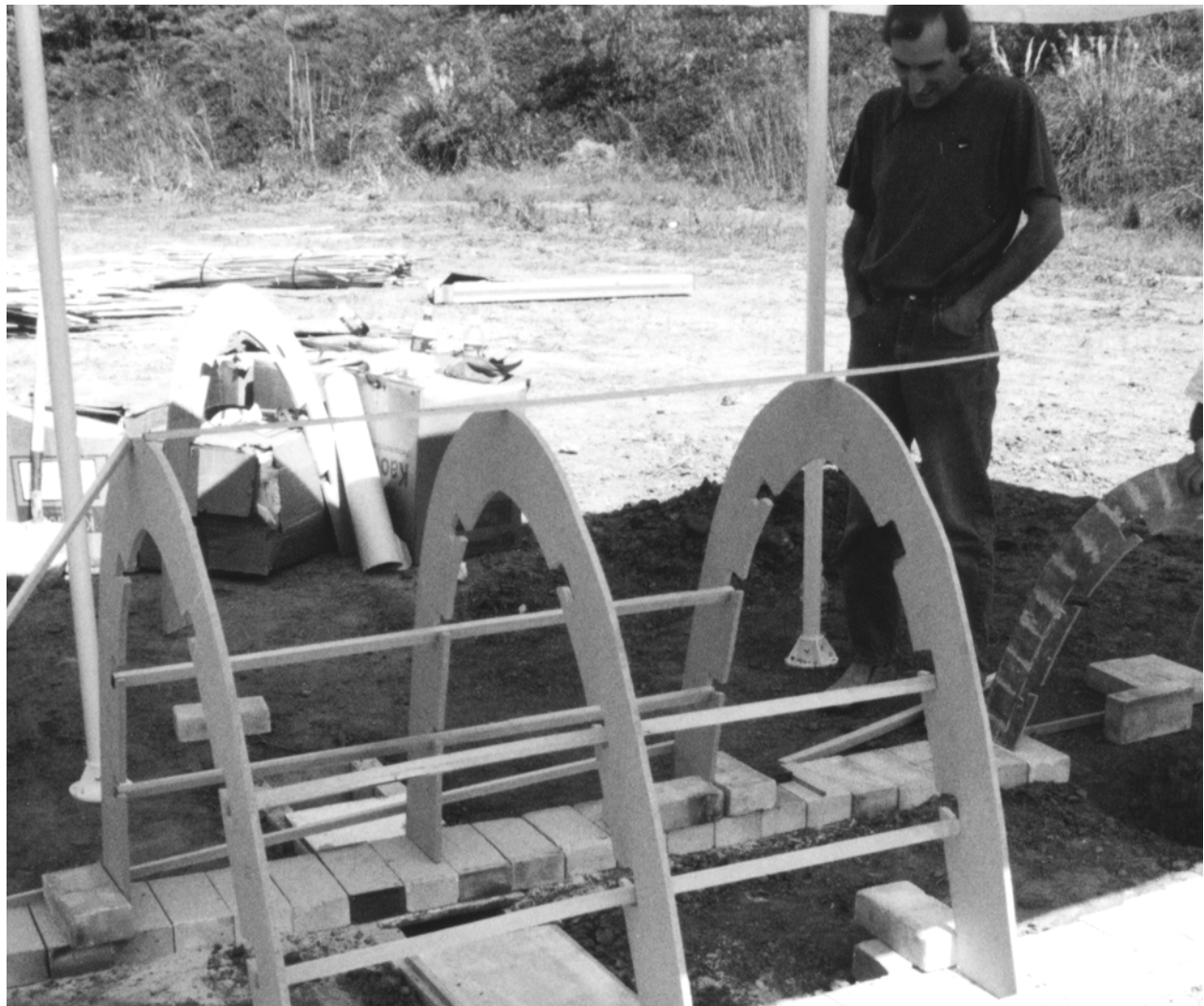
Students learned first-hand how to build a kiln and fire with wood, a process that can be traced back to 6 th century China.
