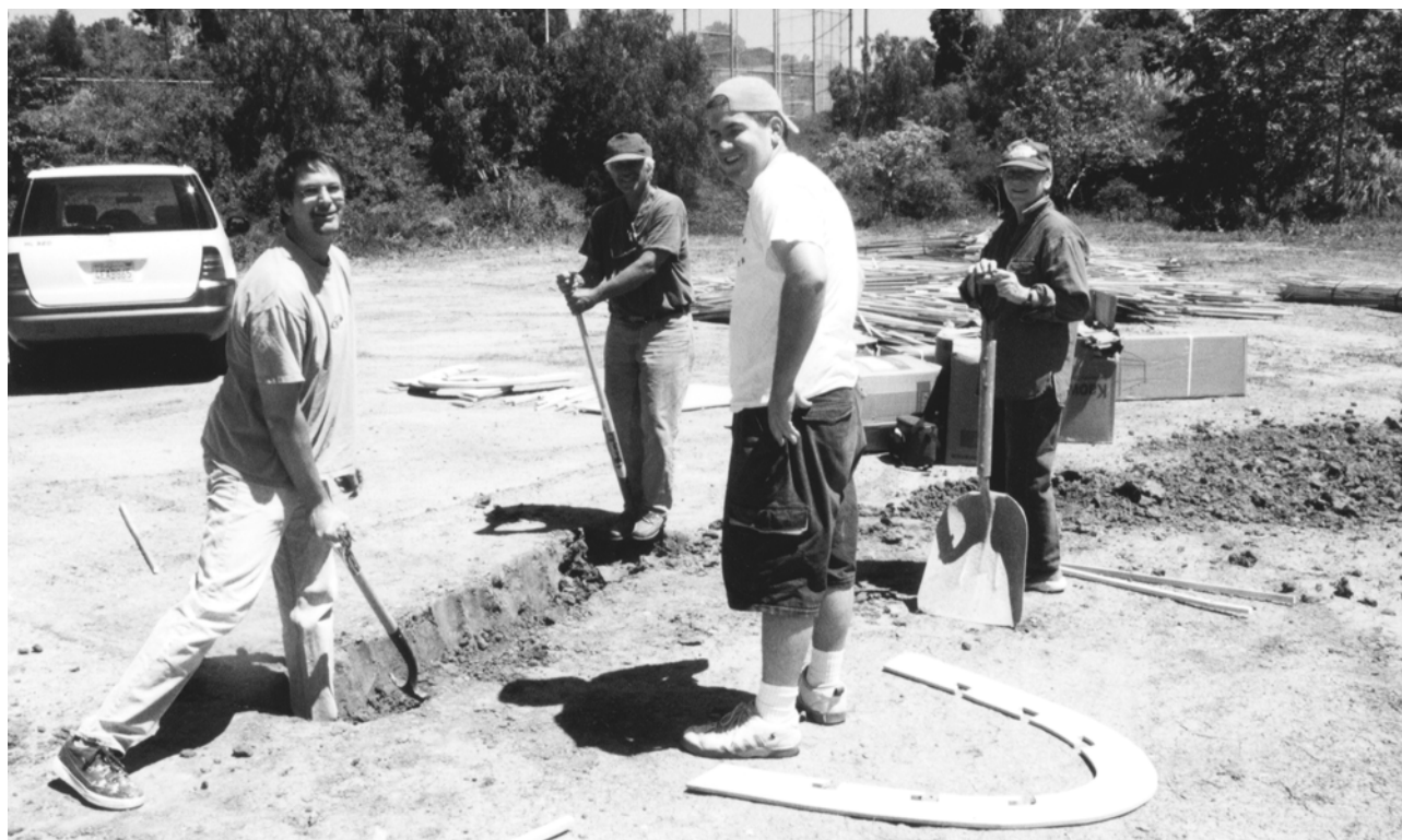
A trench to hold wood ran under the kiln. Two cords of wood were used to fire the kiln, which necessitated round-the-clock attention over a 3-day period.
